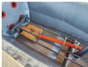
Figure 4 Cable channel (orange color) and wooden block (brown color)
