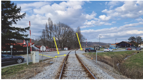
Figure 8 The crossing on the L202 railway line, secured by half-bumpers, with a light-sound measure, has a pedestrian crossing fence. The elements of the road level are poorly integrated into the crossing itself and the existing condition (on a short stretch, up to the yellow dashed line, a greater height difference has been overcome, big “jumps” for BUS and trucks when crossing)
