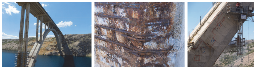
Figure 3 Corrosion of the reinforcement on structural elements of the Maslenica Bridge before and during repair
