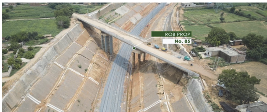
Figure 2 Site Photograph Displaying Bridge Location, Track Crossing, and Deep Cut Ground Profile
