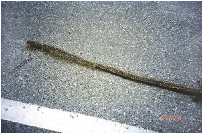
Figure 5 Light Expanded Clay Aggregate (LECA) on the surface of the left part of sealed crack
