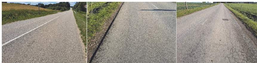
Figure 1 Typical good (left), moderate (middle) and severe (right) pavement condition of the studied low-volume roads
