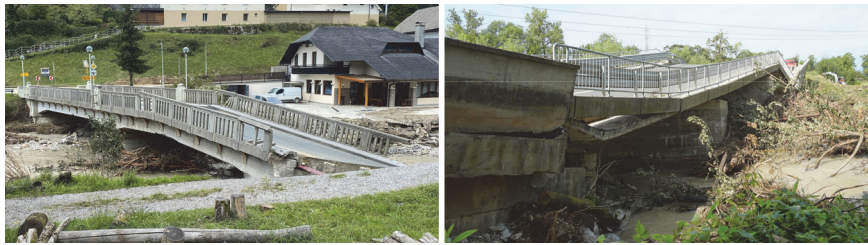
Figure 1 Collapsed bridges in Slovenia after August 2023 floods
