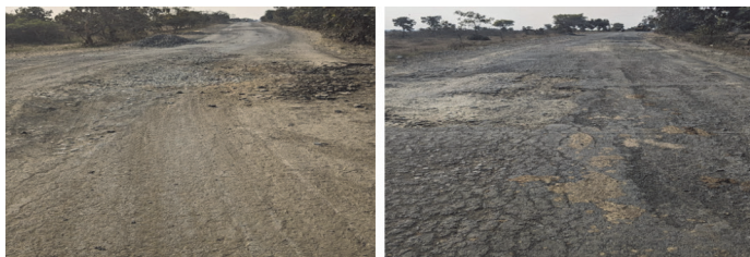
Figure 1 Damaged Low-volume Roads
