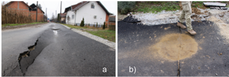
Figure 3 A liquefaction occurrence at the location of N. Drenčina as an aftermath of December 2020 earthquake: (a) deformed road, (b) sand ejecta
