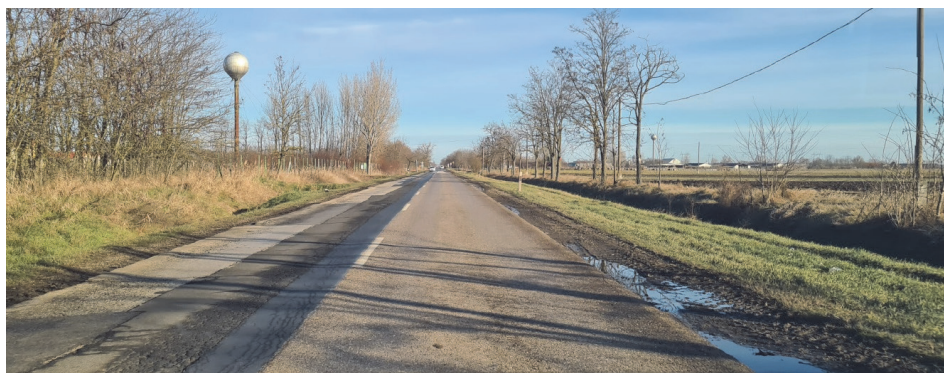
Figure 1 Typical failures of road shoulders - on the right, rutted, too wide shoulder with improper fall; on the left, blown up shoulder (Photo: Zsolt Bencze)
