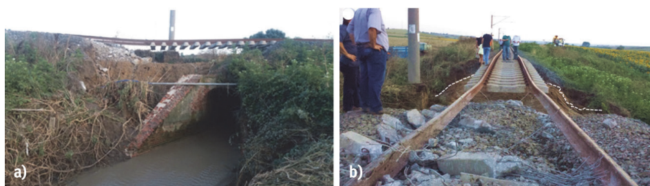
Figure 5 a) Undermined railway track and the (b) collapsed embankment [11]
