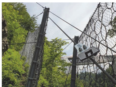
Figure 5 Guard mounted on the support cable of a rock-fall protection structure
