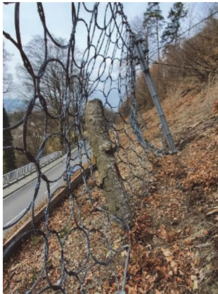
Figure 10 Cutting of a tree trunk after clearing and grubbing of vegetation around the construction
