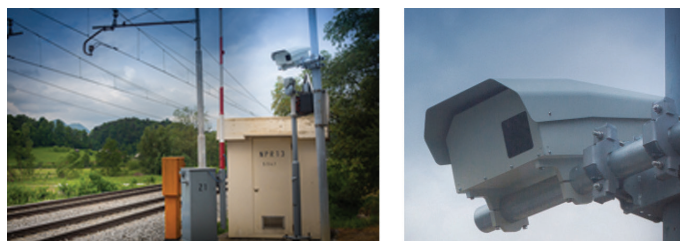
Figure 2 LiDAR sensor installed at the level crossing
