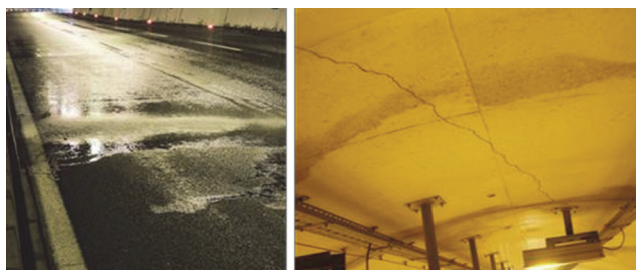
Figure 1 Leakage and cracking in tunnels due to the external forces
