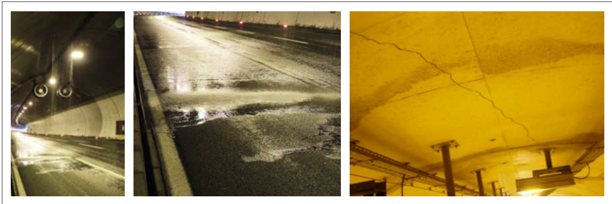
Figure 1 Heavy leaking through tunnel lining and water on the pavement as a consequence influencing traffic safety; cracks on tunnel ceiling [4]
