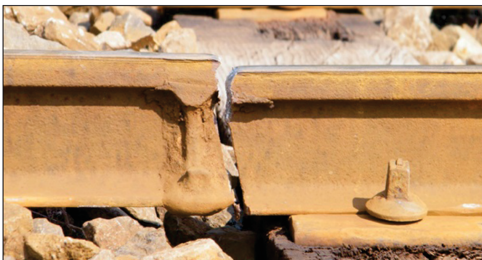
Figure 6 Effects of bad welds
