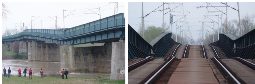
Figure 2 Failure of railway bridge pier in Zagreb, Croatia (31st March 2009)
